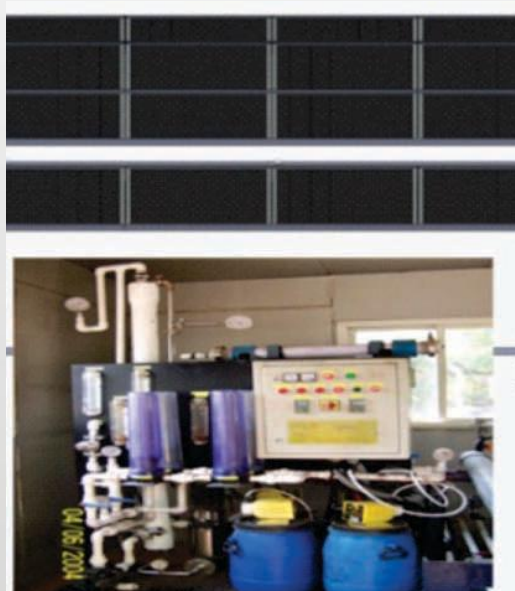
Solar RO Plant
