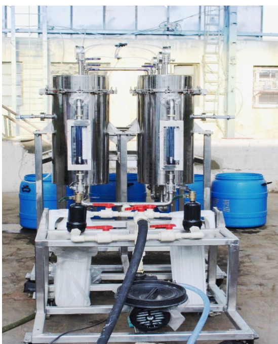
A 15 KLD pilot plant installed at the Heavy Water Plant at Vadodara.
