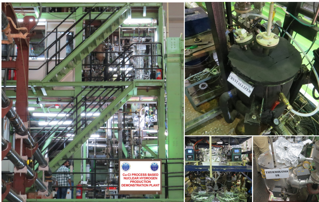
Copper-Chlorine thermochemical cycle pilot plant of BARC coupled with secondary sodium system of FBTR.
