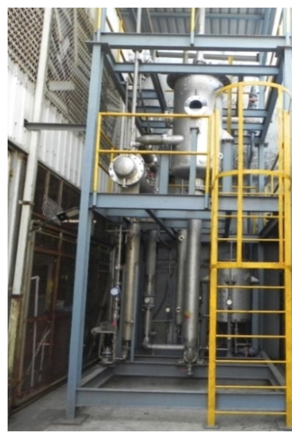
Forced Circulation Crystallizer Unit at BARC.
