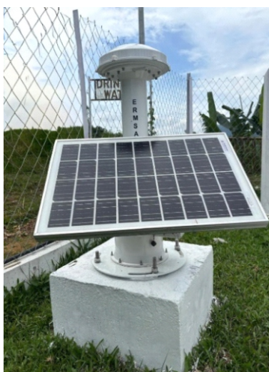
ERMSAT installed in Mizoram.
