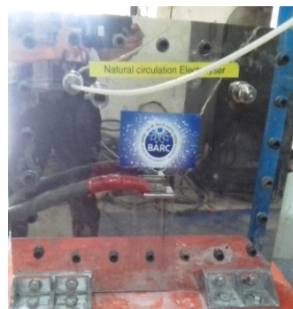
Fig.8: Hybrid natural circulation electrolyser stack under operation.
