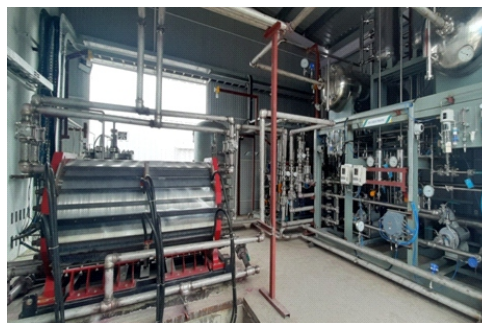
Fig.6: Indigenous 0.5 MW alkaline water electrolyser stack integrated with BOP in collaboration with BPCL at the premises of CIAL, Kochi.
