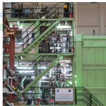
Fig.3: Integrated Cu-Cl-FBTR facility.
