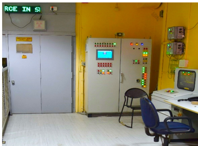
Fig.3: Control room with control panel and SCADA panel of modernized FPI.
