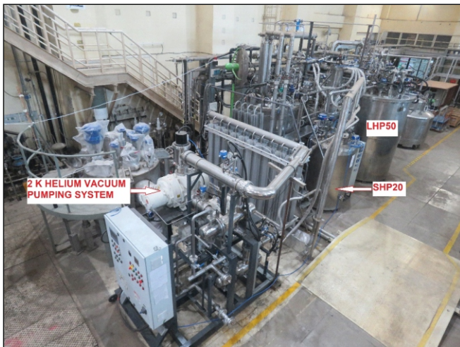
Fig.3: Bird's-eye view of the SHP20 cold box installation along with LHP50 cold box and warm pumping system (WPS).
