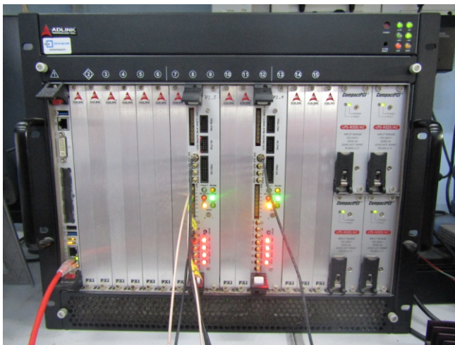
Fig.8: Two LLRF controllers in a cPCI chassis for LEHIPA.
