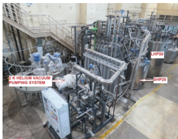
The 2K helium vacuum pumping system
