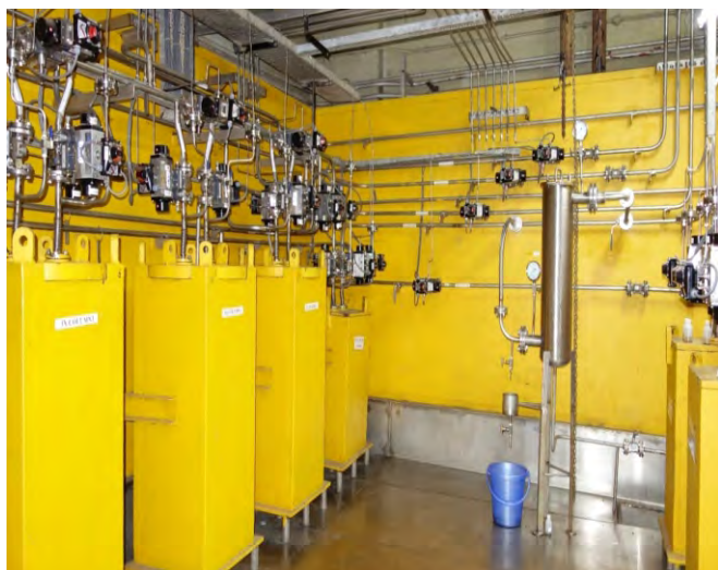
The Effluent polishing system at WIP Trombay.
