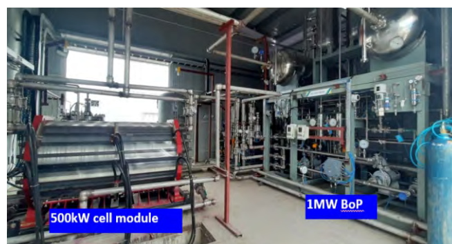
Alkaline Water Electrolyser Plant installed at CIAL, Kochi.
