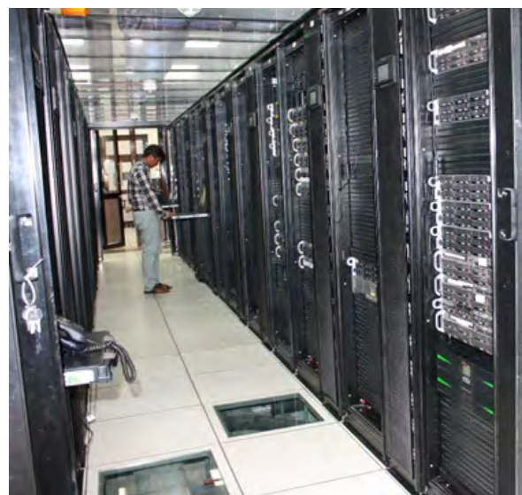
Upgraded MLCC and 15 PetaByte Storage Facility.
