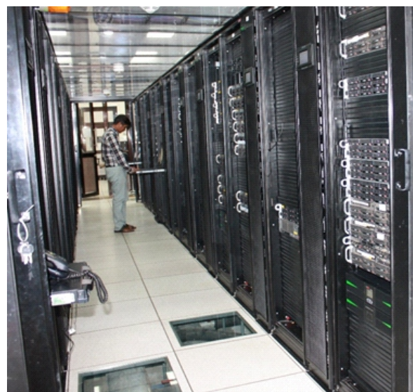
Upgraded MLCC and 15 PetaByte Storage Facility.
