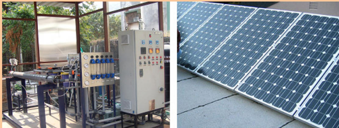
Fig. 5: Community Level RO Plant along with PV Panels at Trombay
