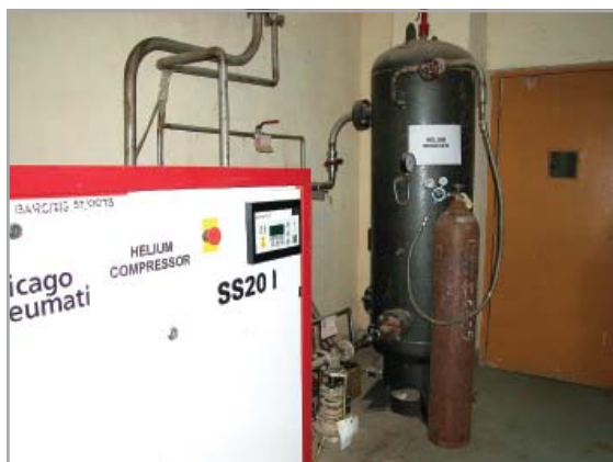
Air compressors modified for helium service are being used for laboratory test set-up
