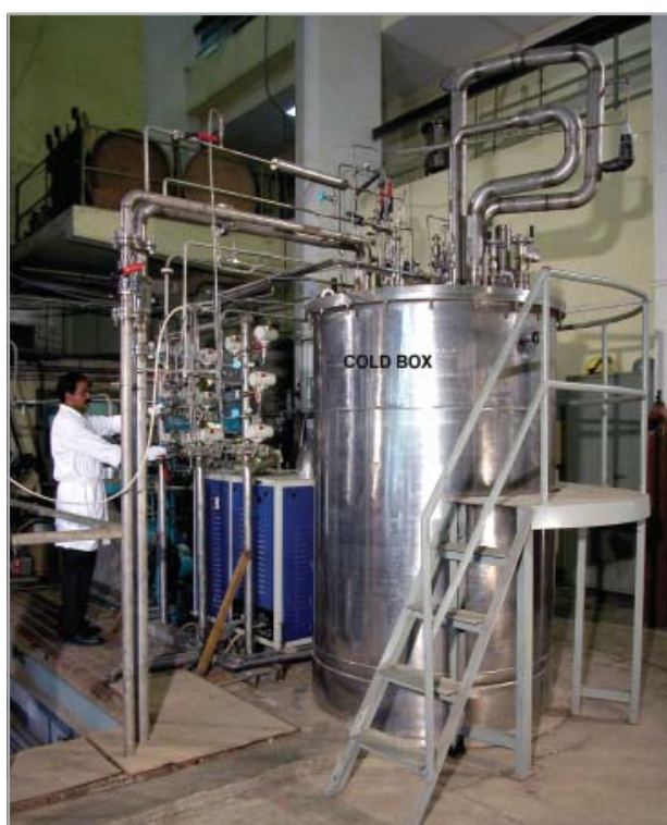
The prototype 1kW at 20K Cryogenic Refrigeration system developed and installed at BARC.
