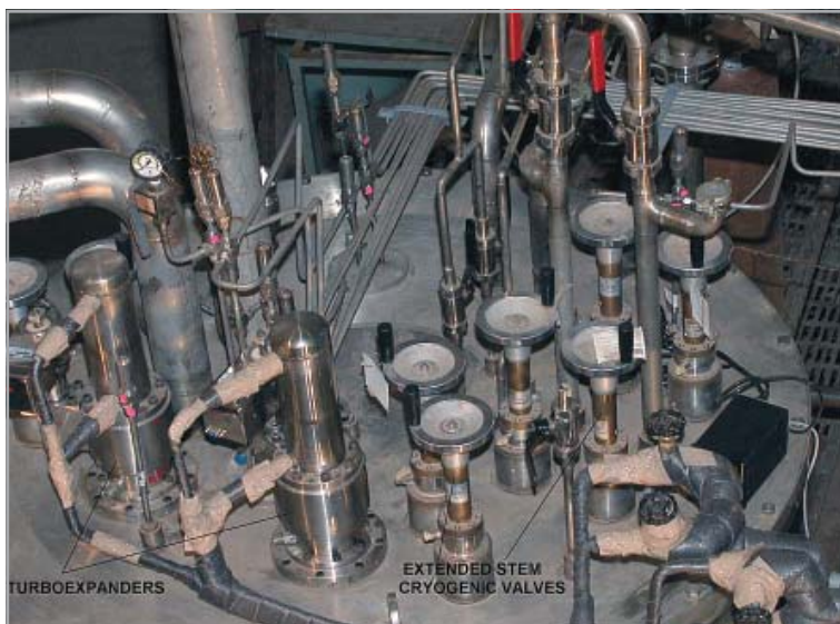
A close-up of the prototype refrigeration system showing turboexpanders, extended stem valves, and external piping mounted on the top cover of the cold box
