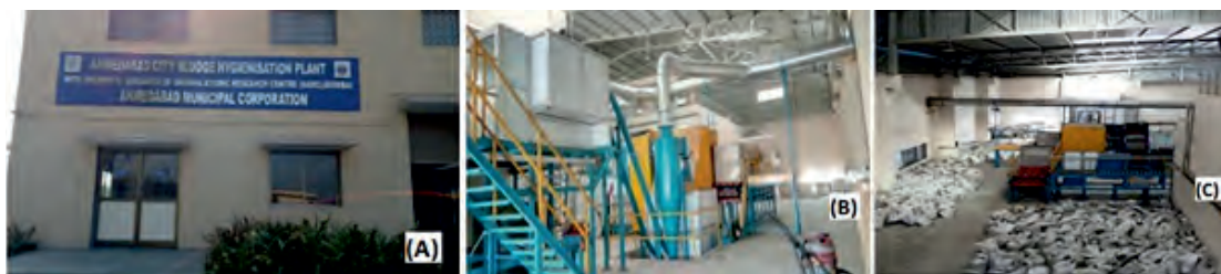
Figure 7: Radiation hygienization plant at Ahmedabad (A) Outside view of the plant (B) Inside view of the plant (C) Processed sludge bags
