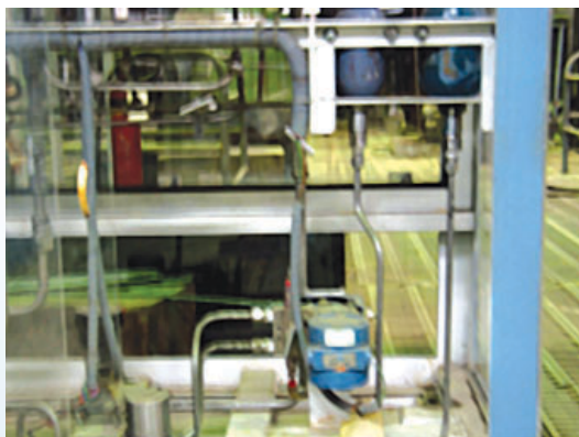
Leak Detector Circuit installed at FMTF of Hall 7
