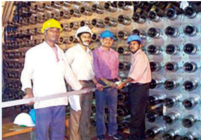
Sag measurement being carried out in TAPS 4
