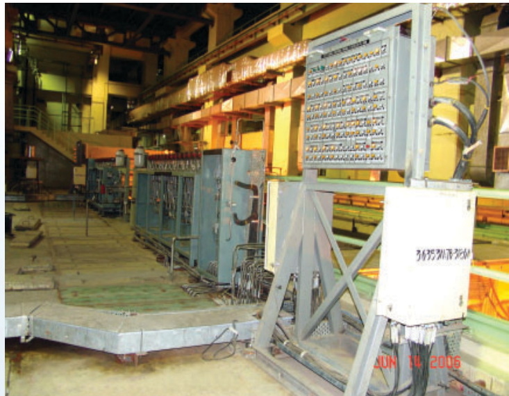
Fig. 6: Water hydraulic valve station
