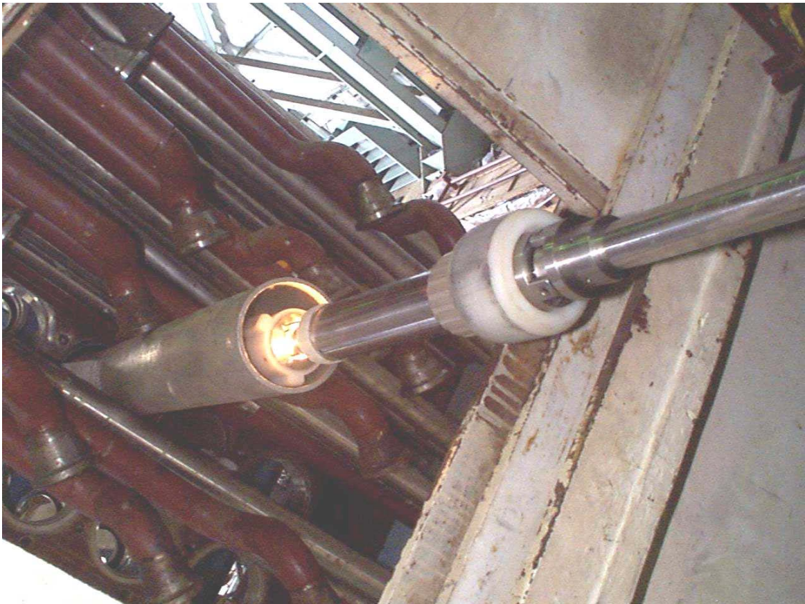
Fig. 7 Camera being inserted into the calandria tube
