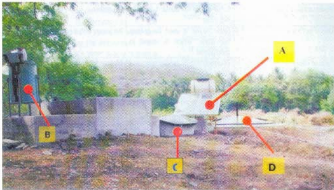
Biogas plant based on kitchen waste
