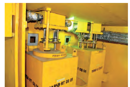
Ion Exchange columns at PHIX System.
