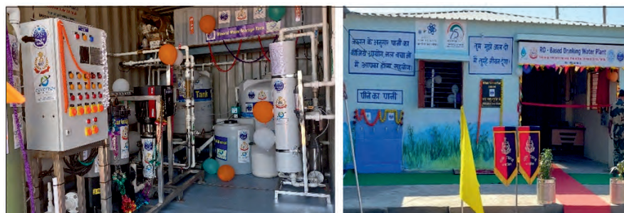
Left to Right: Water purification unit commissioned at Creek BOP, Bhuj, Gujarat; and another at Sandeep BOP, Bhuj, Gujarat.
