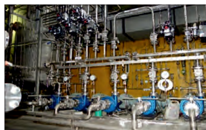
MWPF Raffinate Conditioning and Transfer System at WIP, Trombay.
