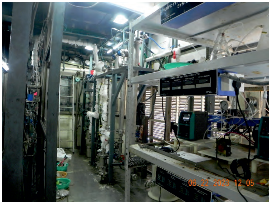
First-of-its-kind integrated closed loop metallic Copper-Chlorine facility in BARC.
