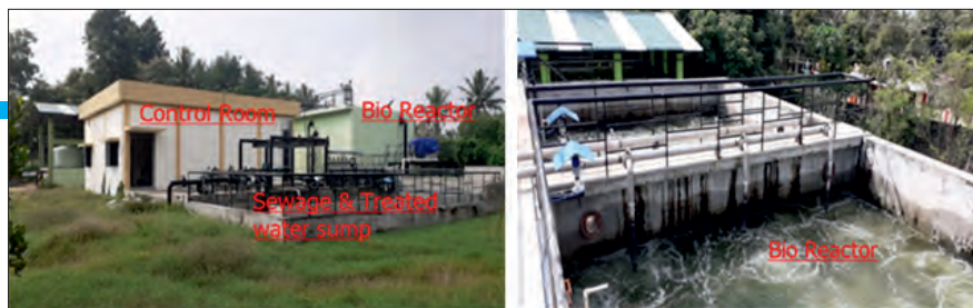
The hgSBR plant installed at Kalpakkam township.
