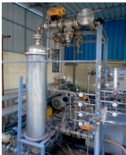
UF system for recovery of water from LL effluent and re-use as process water.
