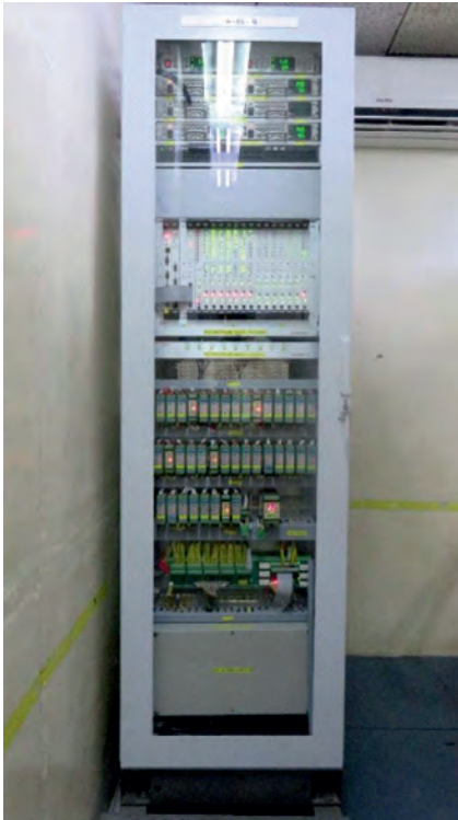
Sub-System-II Panel of ICIS of KAMINI.
