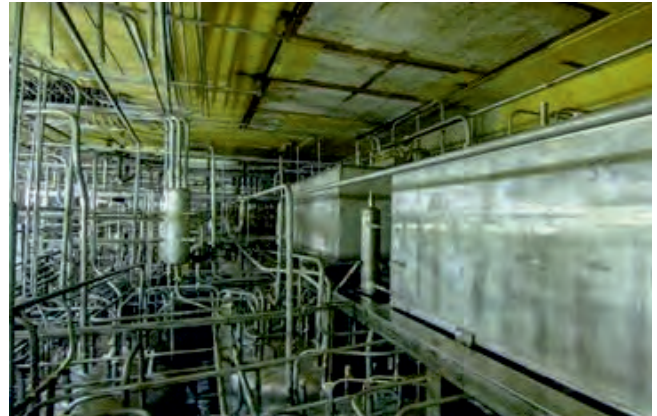
Solvent extraction system for High Level Liquid Waste in WIP, Trombay.
