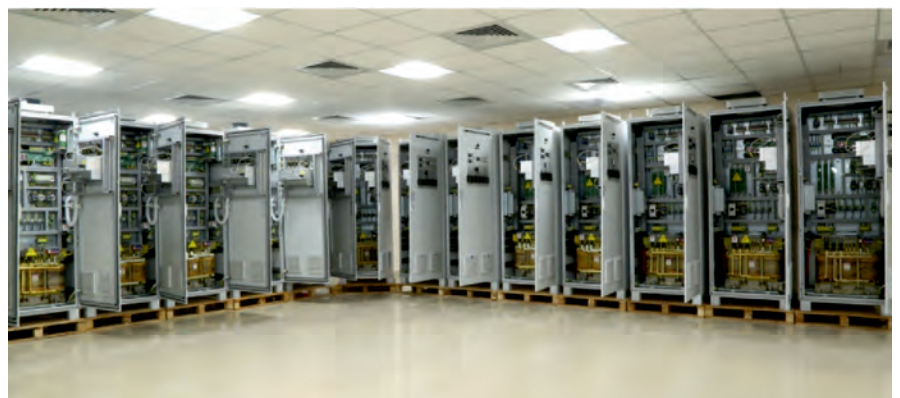
525Amp, 53.5V Power Converters HB.Q11 (35 Nos).
