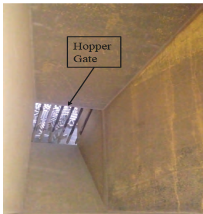
Fig. 6: Internal view of fork-type gate HULL DRUM IMPACT WRECH FIXTURE of hull hopper
