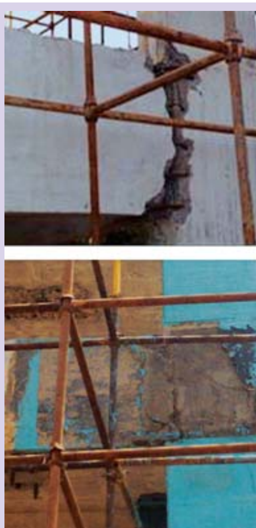
Fig. 6: Failure of beams of as built and retrofitted structure
