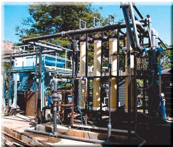
Fig. 5: The ultrafiltration pretreatment plant at the Desalination Division, BARC
