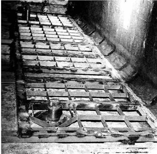
A view of reactor pool wall during lining work showing the Back-up Carbon Steel framework anchored to concrete
