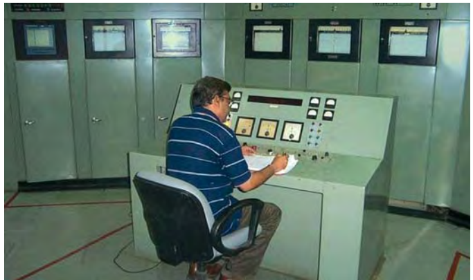
Apsara Reactor Control Room
