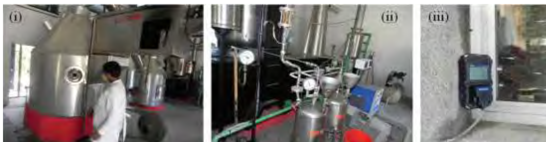
Fig. 2: Photographs of different parts of the chemical incinerator installed at BARC (i) Main combustion chamber (MCC) and Post combustion chamber (PCC) of chemical incinerator, (ii) Feeding vessel, air compressor, spray nozzle, and (iii) Sensor for environmental monitoring
