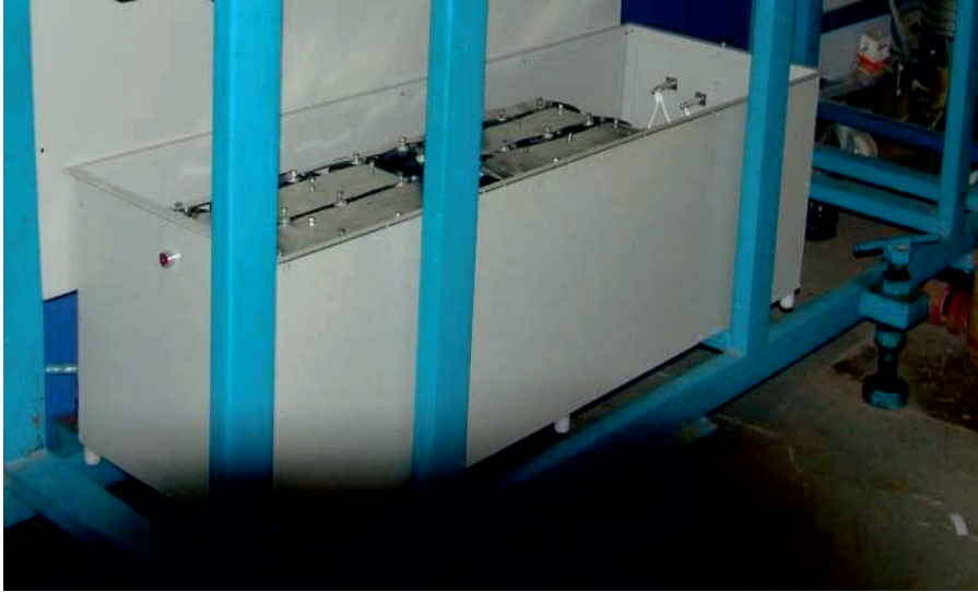
Figure 17.12. 1.1 mF, 6.6 kV capacitor bank.
