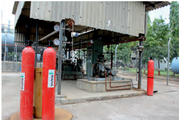
Figure 4: Deuterium gas generation facility at HWP Baroda
