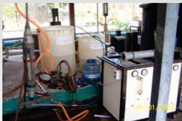
Community Level Water Purification Unit for Iron Removal
