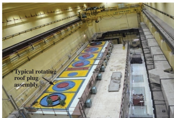
Fig. 3: Hot cell roof with rotating roof plug assemblies
