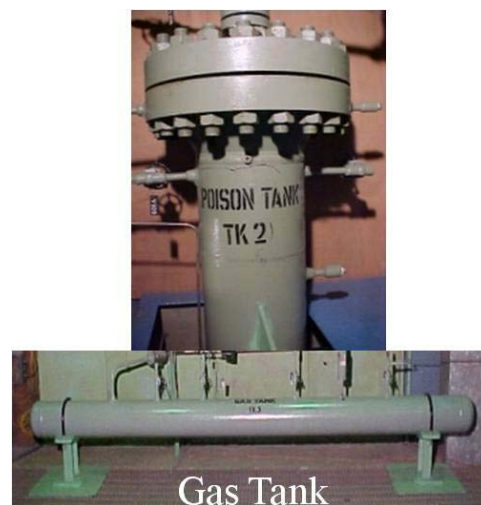
(c) Poison and gas tanks of liquid poison injection system
