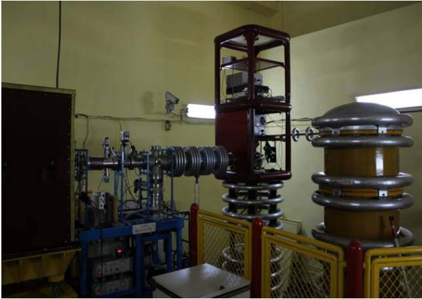
Fig. 2: Purnima neutron generator facility (PNGF)
