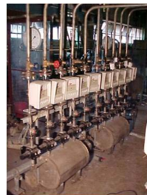
(b) Air injection system
