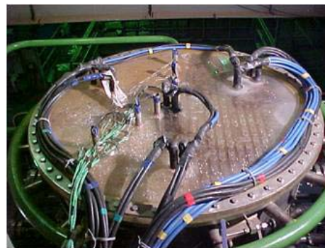
(b) Electrical and instrumentation connection at the top the calandria
