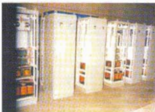
GMRT Motor drive cabinets
