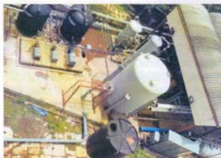
Fig.5 SWRO pilot plant at Trombay
