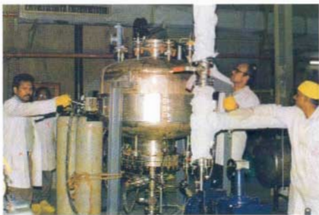
Fig 3 Chemical Preparation Tank (CPT) with the metering pump in front
