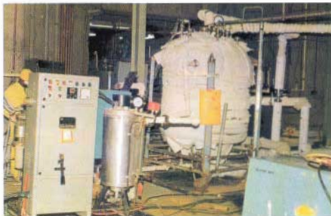
Fig 2 Chemical Addition Tank (CAT) with Electrode Boiler (EB) in front
