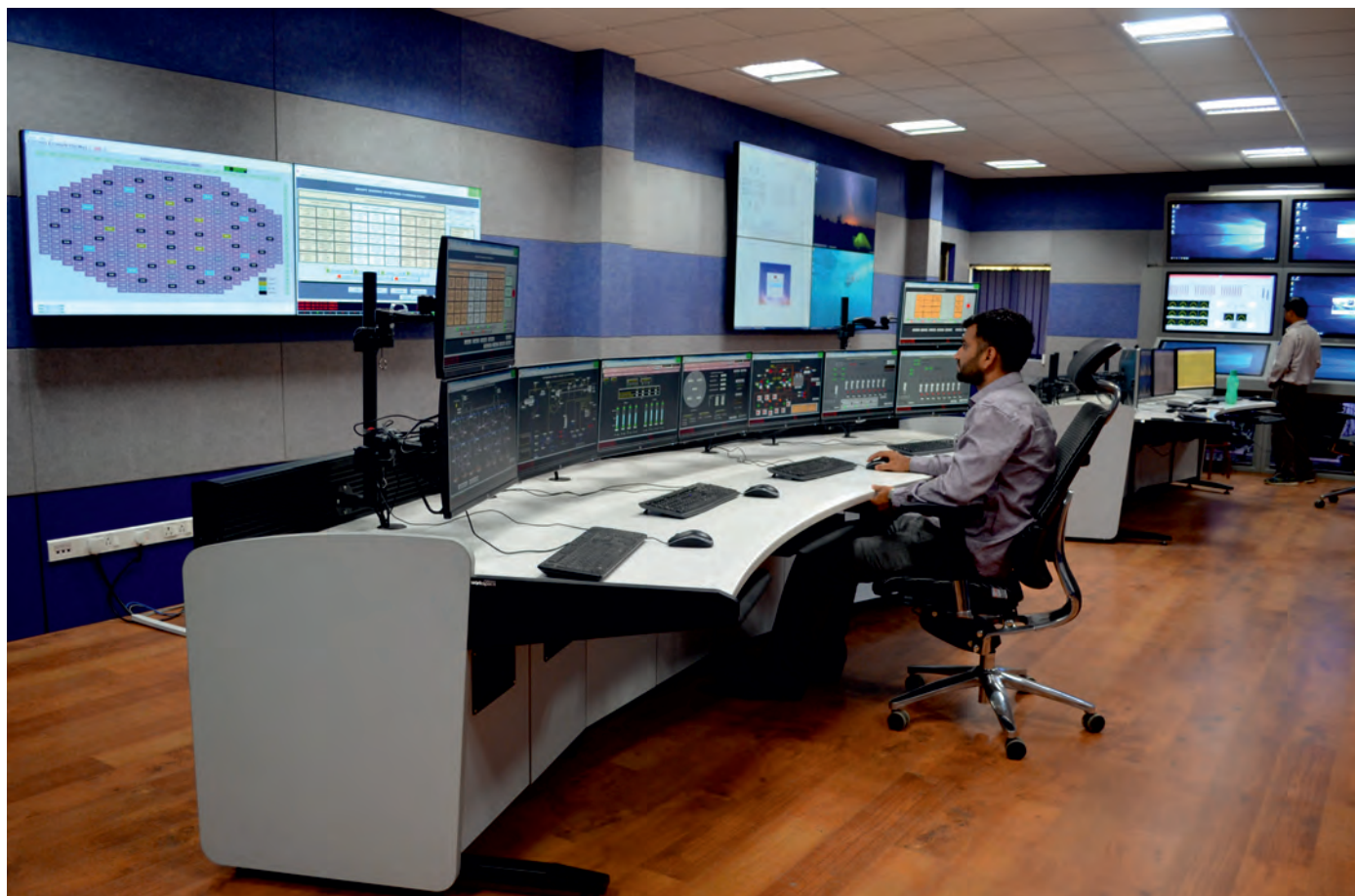
Fig.1. AHWR Simulator Facility in Integrated Test Station at RCnD, BARC, Trombay
