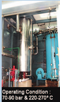
Fig. 8 : Part of HPHT Loop of Leak Test Facility at Jadavapur University, Kolkata
